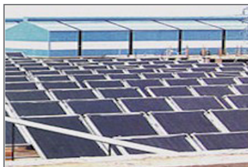
Fig 3.15: Solar Panels to trap solar energy
